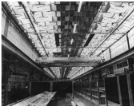
Acoustic absorption treatment showing suspended panels
